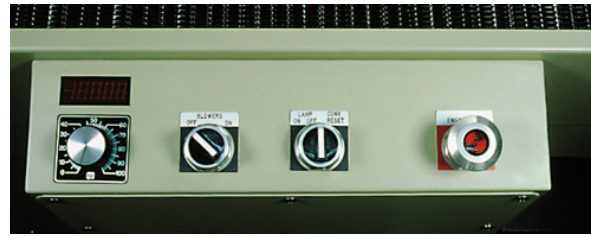
System control panel.
